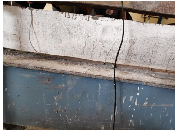
FIGURE 13 CRACKS ON BEAM
